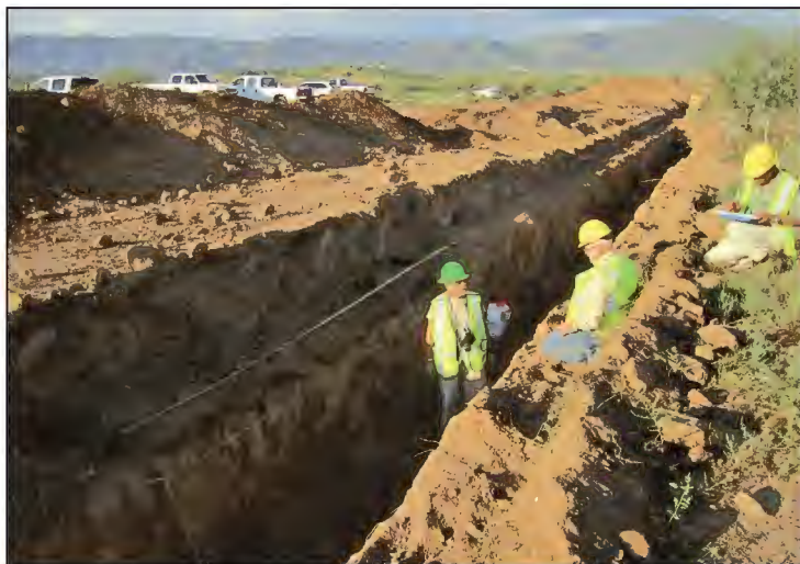
Work is suspended on the discovery of a pithouse. VVAC crews record the site so work can continue.
