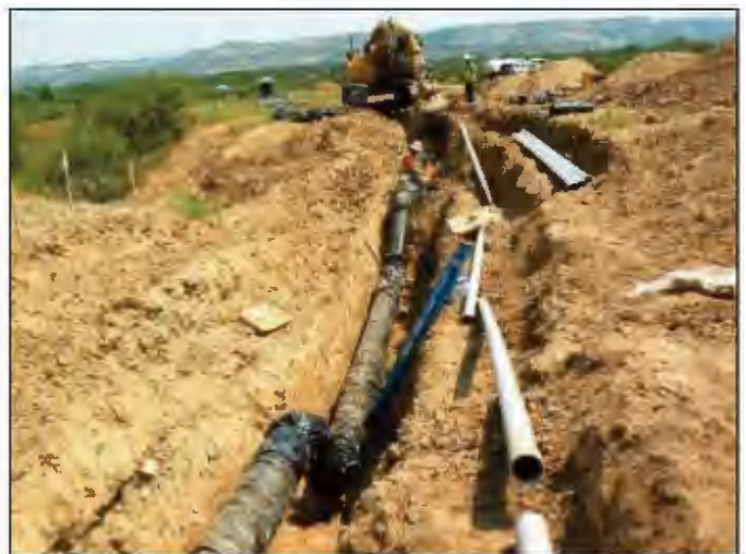
Utilities included the water main as well as conduit for fiber optic cables and electricity.
